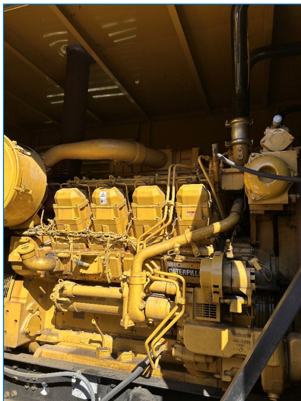
Diesel Engine powering Southern Avenue Plant
